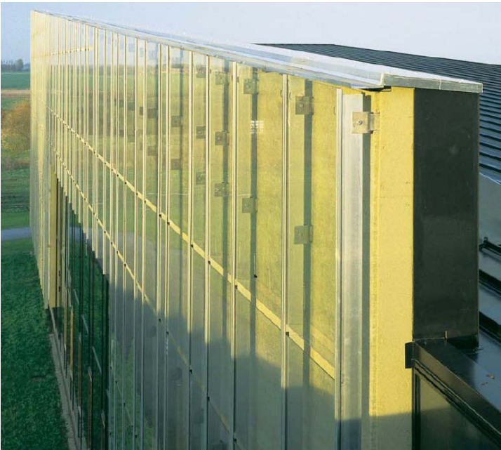
Figure 1 – Open jointed rainscreen on Rockwool/Roxul's Head office in Denmark. Note the open joints in the exterior glass façade allowing for moisture egress and exposure to UV light. Joints in the glass façade are approximately 4" wide. More information including actual current exterior and interior temperatures can be found at; http://www1.rockwool.com/environment/building2k/frame_set.htm
